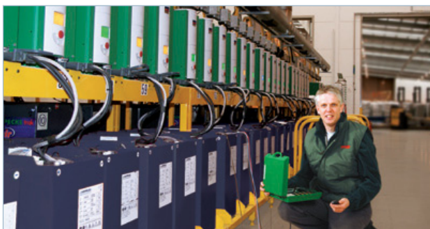
PC-controlled data exchange in a charging station
